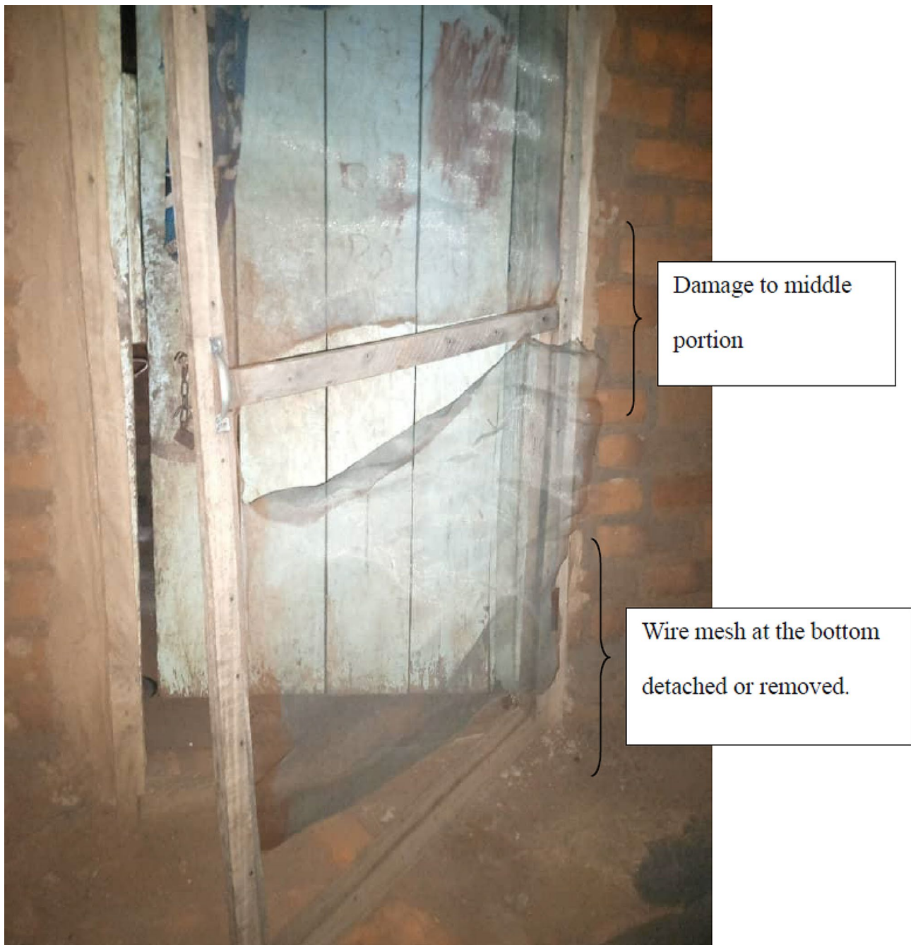
Fig. 3 Damaged door screen showing the portions that were damaged the most
