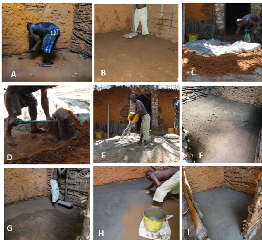
Fig. 2 Installation of the low-cost floor. A) Excavating the existing surface, B) Compacting the soil, C) Adding cement to local subsoil (1 part cement with 9 parts soil), D) Mixing cement with sub-soil, E) Adding water to the mix, F) Cement-stabilized soil laid on top of the compacted soil, G) Compacting the cement-stabilized soil, H) Spreading the “nil” finish (cement/water slurry), I) The completed floor
