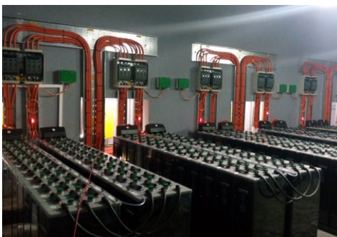
The solar battery backup system at the icipe Thomas Odhiambo Campus, Mbita, on the shores of Lake Victoria, which will supply power during the night for about five hours.
