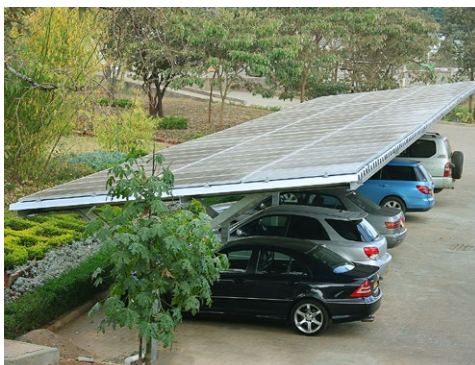
A total of 136 solar photovoltaic (PV) modules have been fixed on carports in both icipe campuses.
