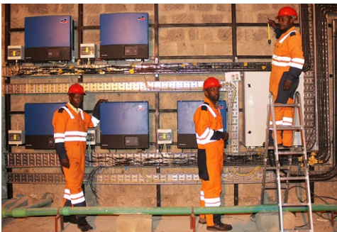
Technicians from Solar Century installing solar inverters, one of the components of the solar PV plants.
