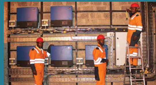
Technicians from Solar Century installing solar inverters, one of the components of the solar PV plants.
