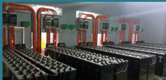
The solar battery backup system at the icipe Thomas Odhiambo Campus, Mbita, on the shores of Lake Victoria, can supply power during the night for about five hours.
