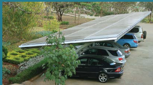
A total of 228 solar photovoltaic (PV) modules have been fixed on carports in both icipe campuses.
